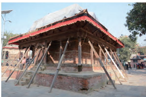
Fig.2-28 Kageshwar temple whose upper floor was collapsed
