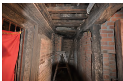
First floor: Slight damage
