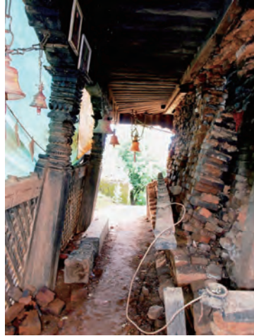
Fig.3-16 East side brick wall. The wall is visibly inclined to the west, the outside dātiapā bricks have fallen down
