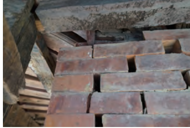
First floor: Periphery wall joint damage
