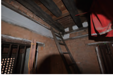
First floor: Inner periphery wall peeling plaster and joint damage
