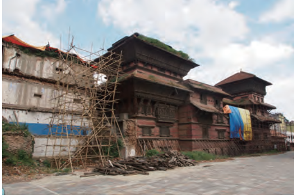
Fig.2-1 Basantapur Bhawan, whose 7th to 9th floors were collapsed
