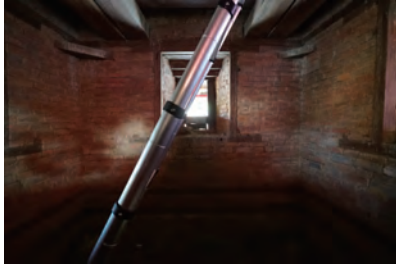
Third floor: Slight periphery wall damage
