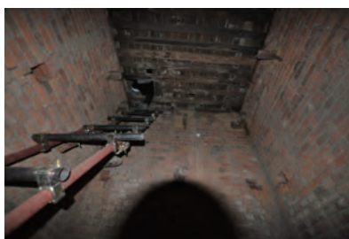
Second floor: Slight inside wall damage
