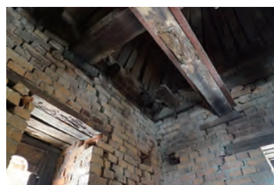
Third (top) floor: Crack at roof beam cut-out (2)
