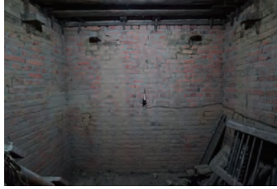
Second floor: Slight inner-periphery wall damage
