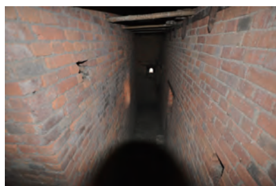
Second floor: Slight inside and outside wall damage
