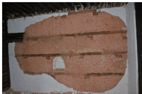
Fig.2-14 Some timber was exposed from inside the wall
