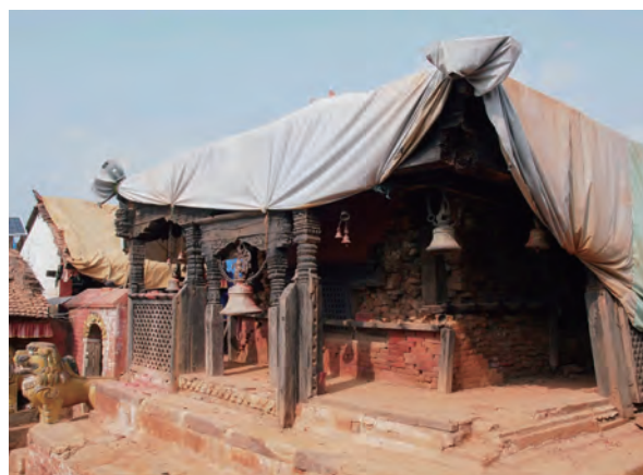
Fig.3-14 Outside view of Bhairab Temple. The corner pillar has fallen down, but the building has not collapsed completely
