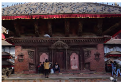
First floor: Slight damage
