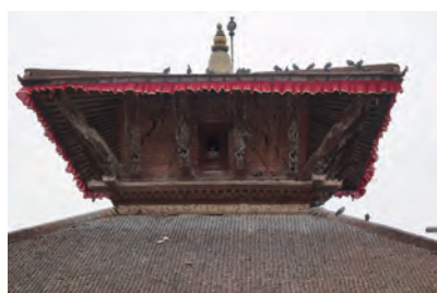
Third (top) floor: Brick wall damage
