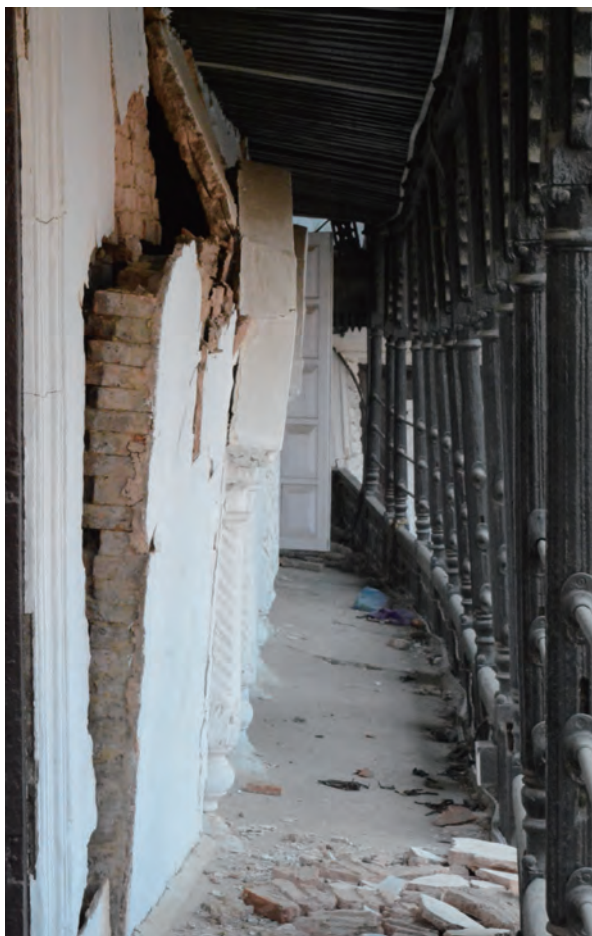
Fig.2-26 Damage situation at the veranda on the second floor of Mohan Chok
