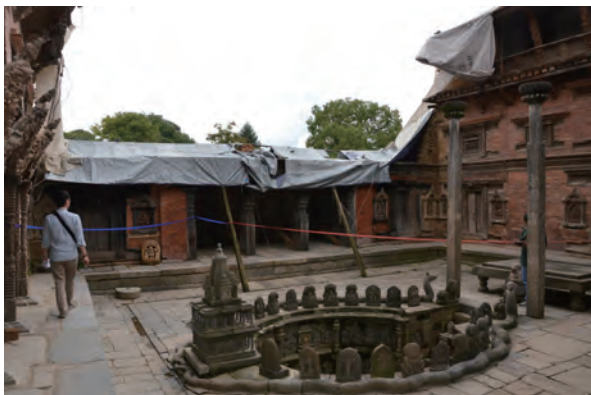
Fig.2-3 Collapsed east-wing of Sundari Chok
