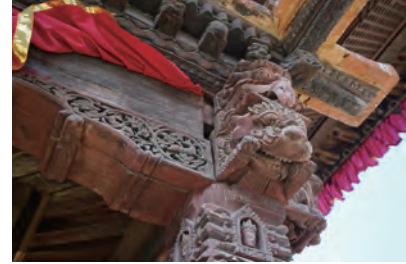
Fallen timber beam
