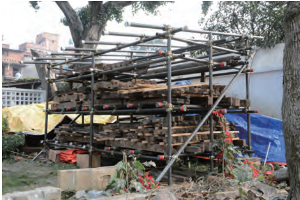
Fig.5-10 Storage condition of the caved members
