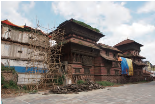
Fig.2-24 Damage situation of the south of Nasal Chok and Lohan Chok
