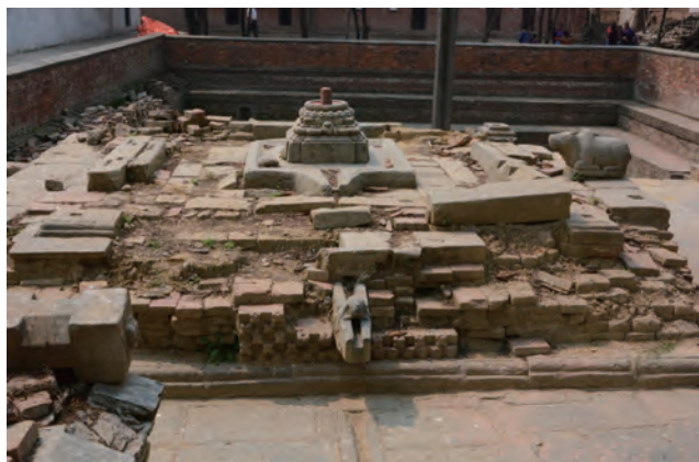
Fig.5-1 Foundation of collapsed Shiva Temple
