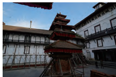
Adjunct tower: Heavy damage
