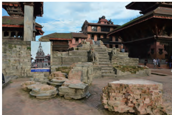
Fig.2-5 Basara Devi (Completely collapsed)
