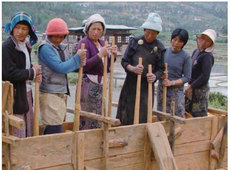
伝統的な版築工法による民家の新築工事 Construction work on a rural house using traditional earth ramming techniques
