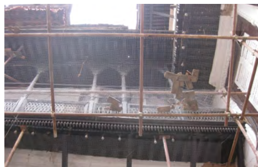
Fig.3-1-23 Tiles felled from the roof above Hanuman gate
