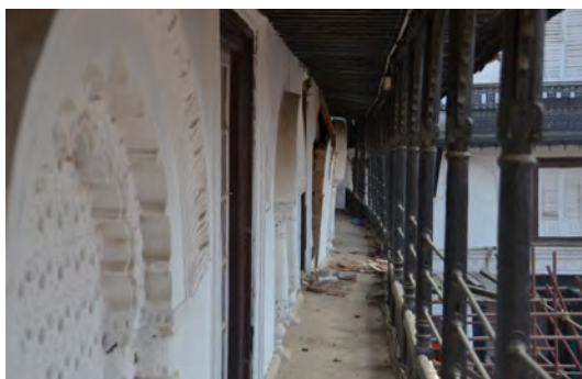
Fig.3-1-14 Damaged condition of the west balcony on the third storey of the west wing of Mohan Chok
