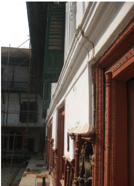
Fig.3-1-18 Deformation condition of the east side of the west wing of Mohan Chok
