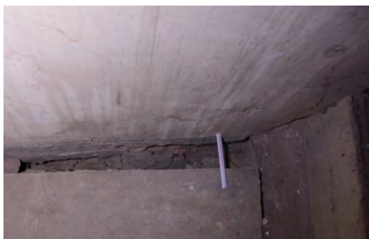
Fig.3-1-22 Gap between the second floor of Hanuman gate and the outer western wall
