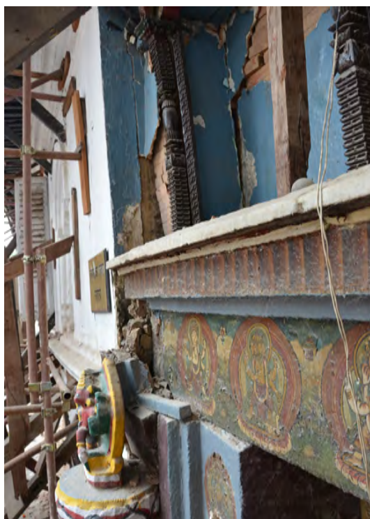
Fig.3-1-20 Damage condition of the upper part of Hanuman gate
