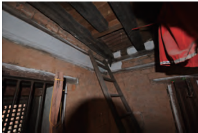
1層内周壁漆喰剥落、目地被害
