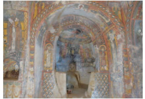
ウフララ渓谷における壁画保全状況調査 Condition survey of a mural painting in Ihlara Valley.
