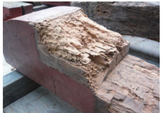
シバンムシに被害された部材 Wood member damaged by anobiid
